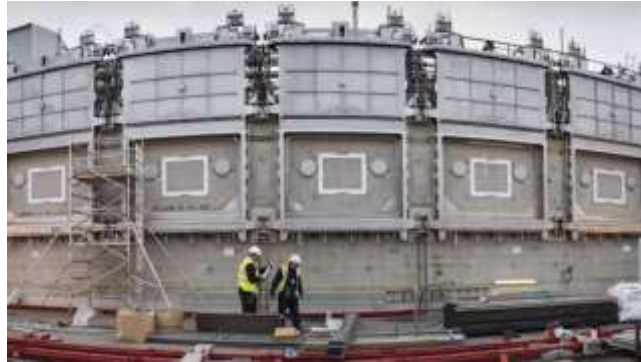
Figure 3: Pile Fuel Cladding Silos (PFCS). This picture shows the external view of one of UK's legacy nuclear storage facilities commissioned in the '50s. The silos house intermediate level waste at the Sellafield sites.
