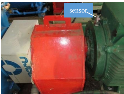
Fig. 6. Vibration sensor mounted on the motor
