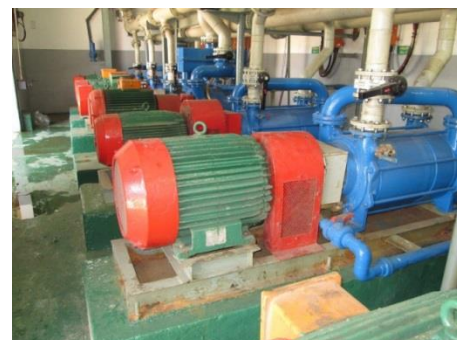
Fig. 4. Centrifugal pump set-up
