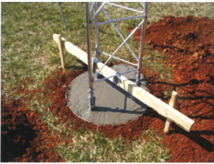
The base of the instrumentation tower.
