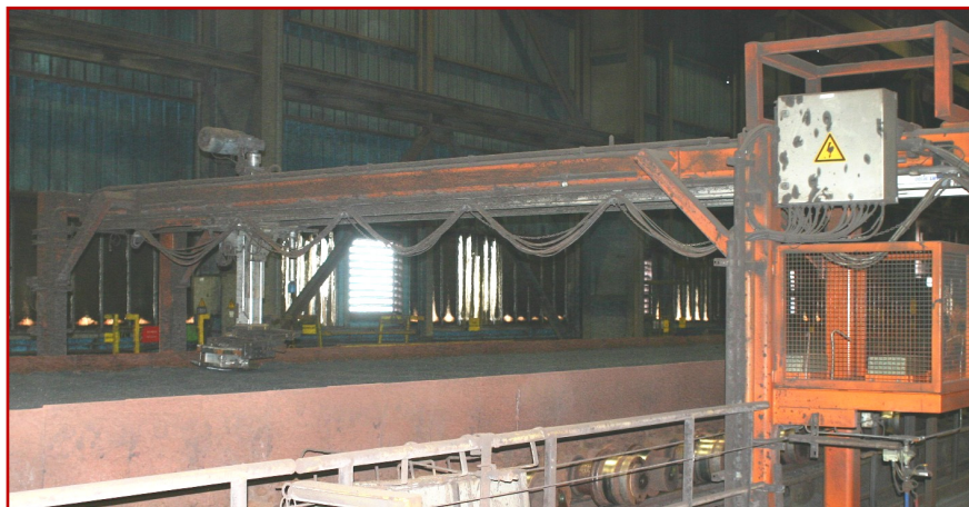
Figure 7: SuPerMagnag system installed on sinter strand SIFA2 at ArcelorMittal Gent
