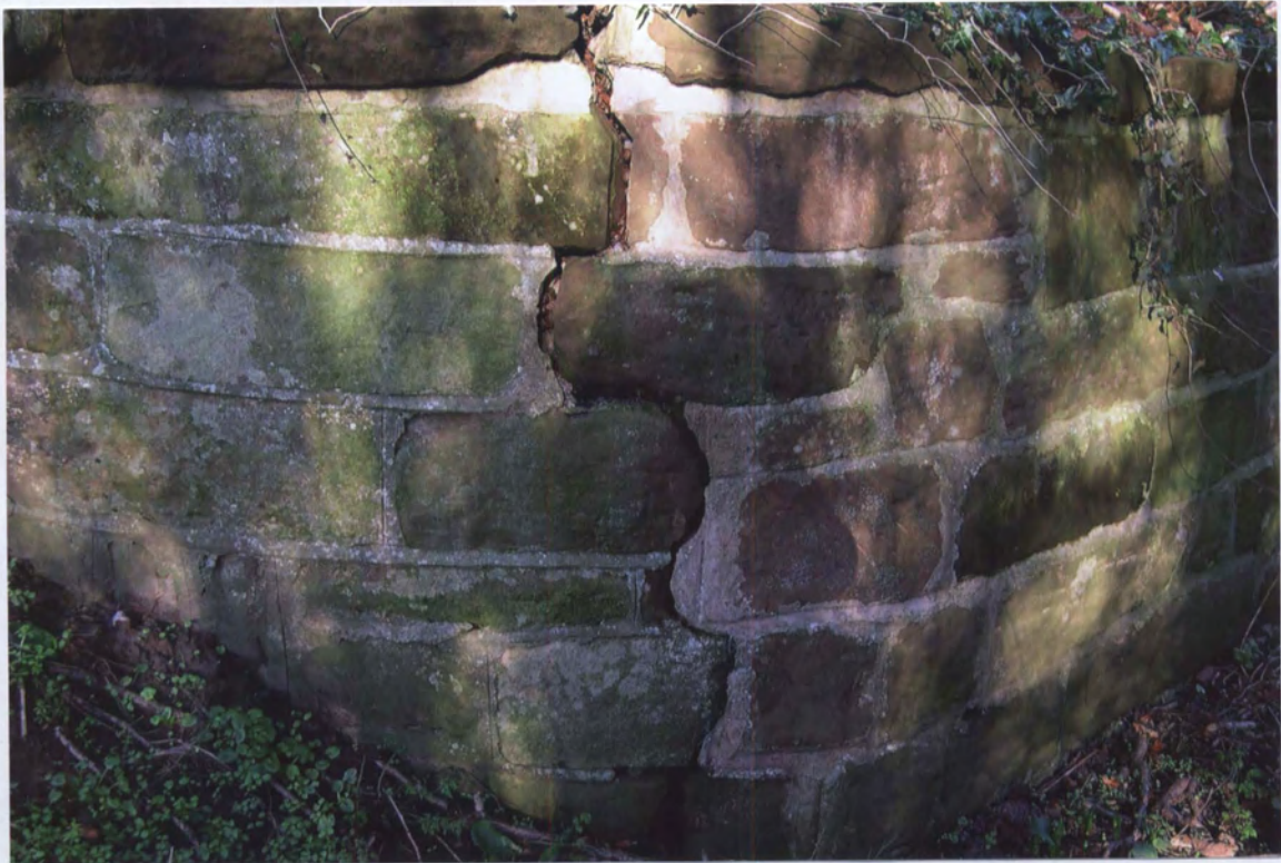
Under pressure: the south-west corner of the churchyard wall, viewed from the trackway.
