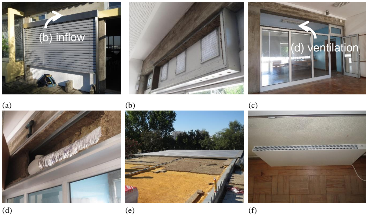
Figure 15 – Prototype interventions: (a) exterior blinds; (b) naturally filtered inflow through the envelope; (c) partition wall; (d) ventilation system - forced airflow to the circulation zone; (e) roof insulation; (f) electric heating system.
