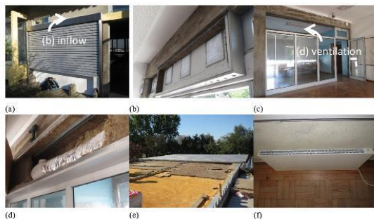
Fig. 6. Prototype interventions: (a) exterior blinds; (b) naturally filtered inflow through the envelope; (c) partition wall; (d) ventilation system - forced airflow to the circulation zone; (e) roof insulation; (f) electric heating system.
