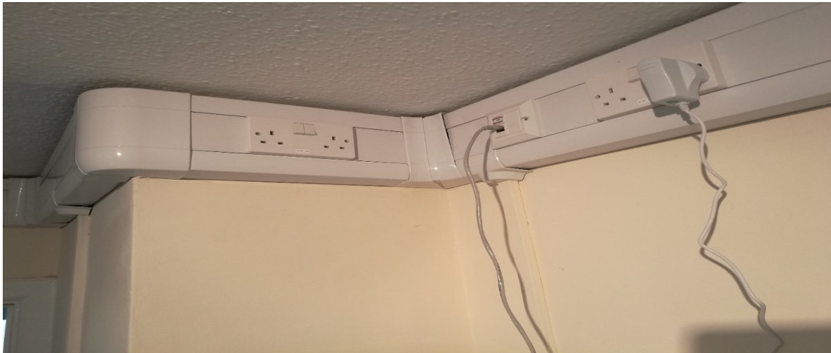
Figure 5. 2 Ethernet ports and power socket in a corner of a room.
