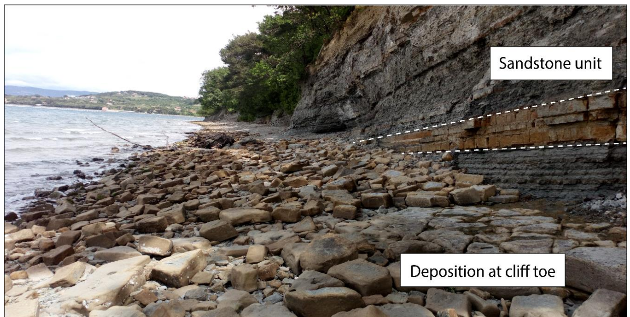
Figure 5.27. Accumulated block deposition at the cliff/platform interface resulting from discontinuous sandstone strata susceptible to block detachment (Punta Grossa, Slovenia). Note the distinct consolidated sandstone strata within the Flysch cliff.
