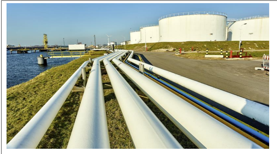
Figure 2.2 Petroleum products pipeline infrastructure.
