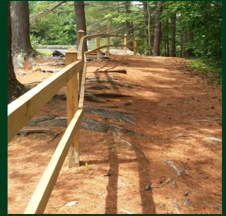
Fence at Runaround Pound built by Nathan Abbott as his Eagle Scout Project 2019
