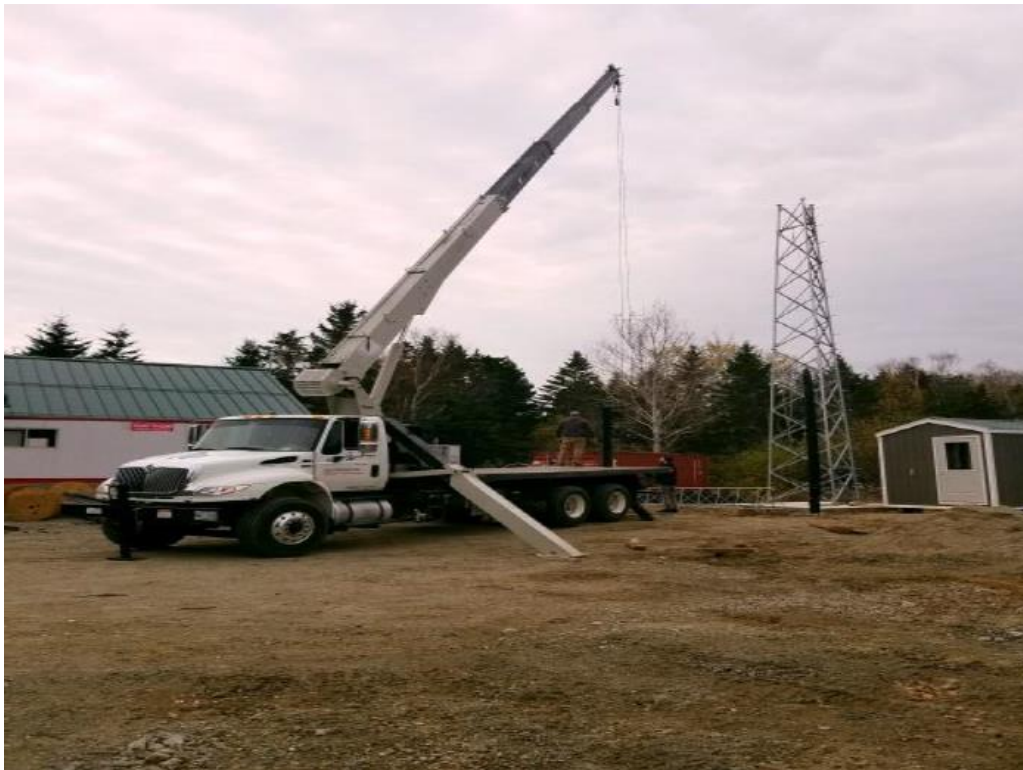
Islesford Tower Build on Town property, next to fire station (Mark Ouellette)
