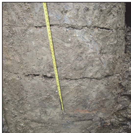
Figure 9 Cracks on pile after unloading from T_{max} = 360.0 kN
