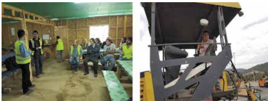
Figure 3. Meeting with the asphalt pavement team (left) and installation of GPS (right)
