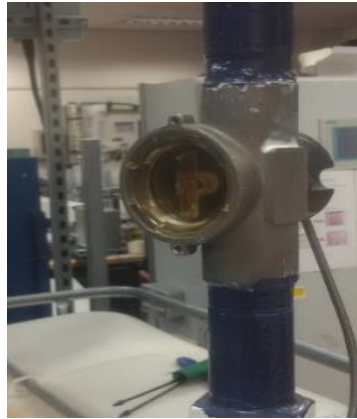
Figure 6-7 Electronic flow sensor in the pipeline
