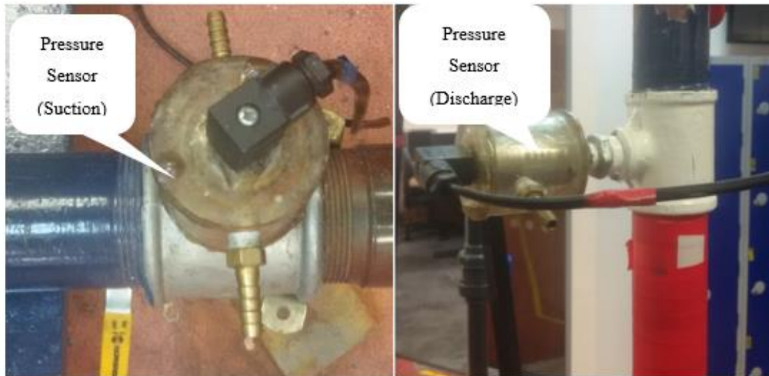
Figure 6-9 Pressure transducers installed at the pump inlet and outlet
