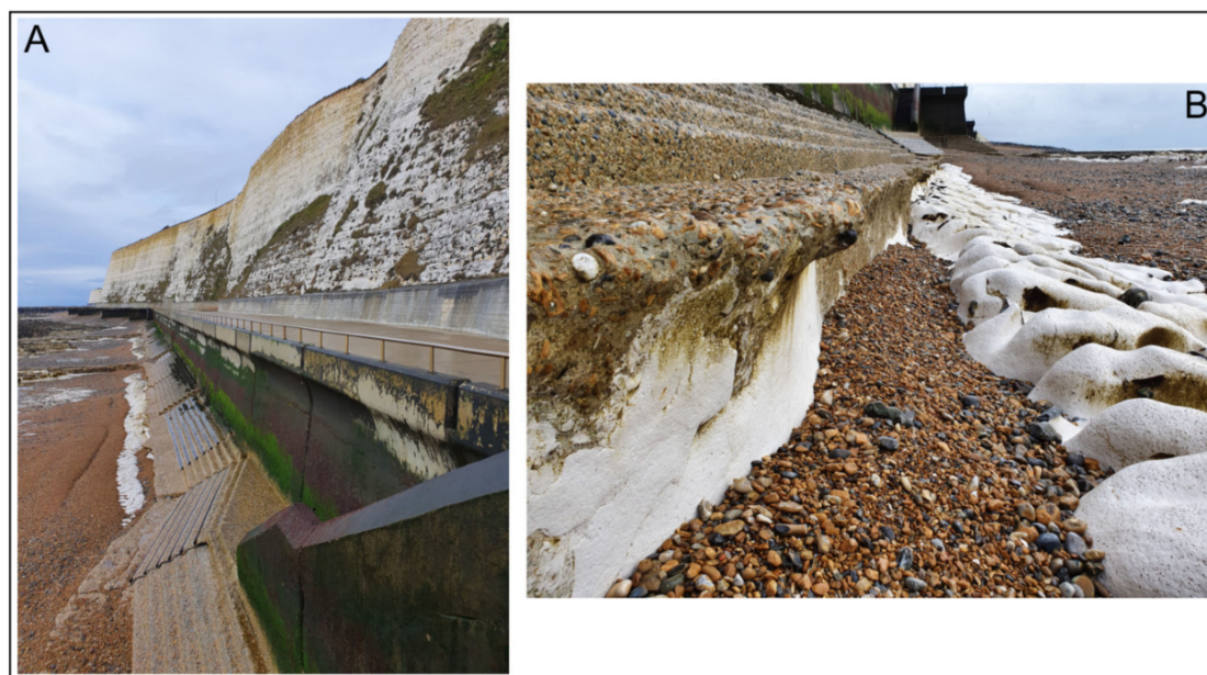
Figure 7. Undercliff Walk in Saltdean. Photograph (A) shows the splash wall, undercliff walk, seawall with small steps and the shingle beach in front of the steps. Photograph (B) presents part of the seawall directly on the shingle beach. Downwearing and erosion at the seawall steps have exposed the base of the seawall foundations and the underlying chalk. The bottom step has a slightly concave shape from continuous wave erosion.
