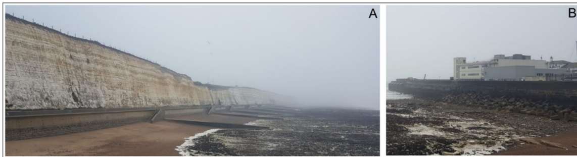
Figure 6. Roedean site at low tide. Photograph (A) showing the view looking east, visible groynes in the distance and sediment accumulating in between, with a chalk platform in front of the sediment. Photograph (B) looking southwest, showing the end of the Marina and a rip-rap shore protection in front.
