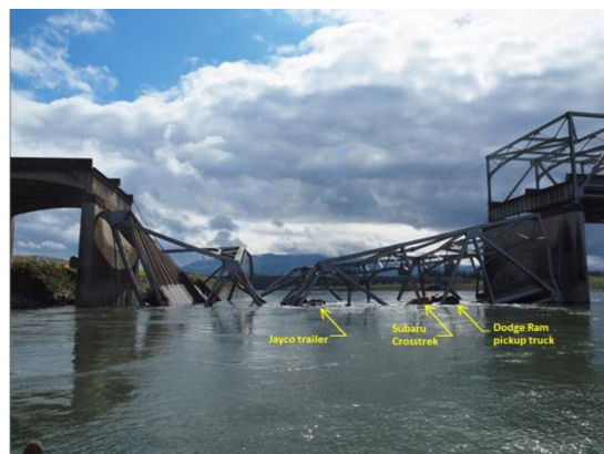
Figure 10. Collapsed Bridge Span. Reprinted from “Collapse of the Interstate 5 Skagit River Bridge,” NTSB, 2013, p.12
