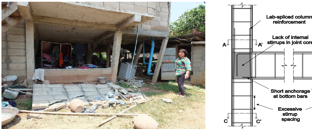
Figure 1 (a) Building partial collapse during the 2014 Mae Lao earthquake (Chaing Rai, Thailand) due to failure of exterior beam-column joints, and (b) typical substandard detailing of beam-column joints in Thailand (adapted from Imjai et al. [6]).
