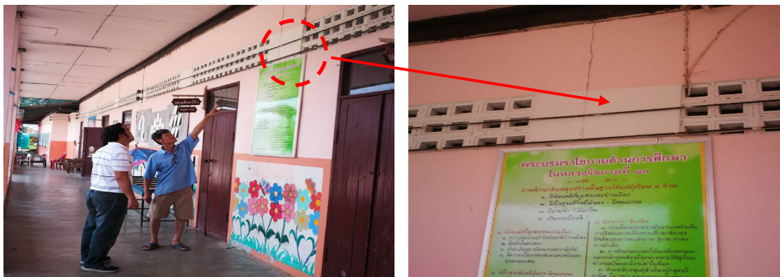
Figure 4 Visual inspection of damaged building performed during phase 1 (photo no. F-01).
