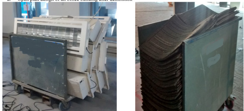
b. Demolished elements placed into wheeled bins (left: lighting fixtures, right: floor carpet)
