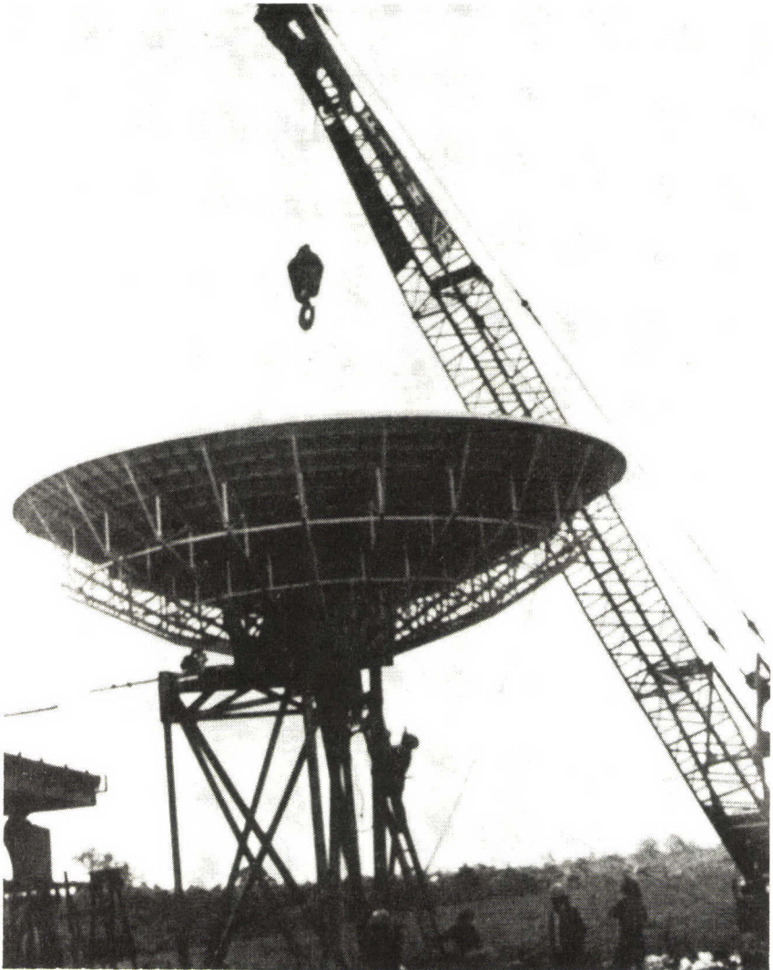
FIGURE 10 32-FOOT DIAMETER PARABOLIC COMMUNICATIONS SATELLITE ANTENNA UNDER CONSTRUCTION AT CIBINONG MASTER CONTROL STATION
