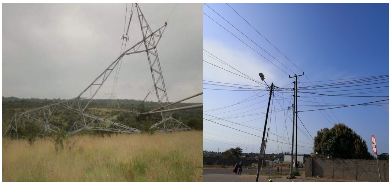
Figure 4: Vandalised power tower (top) and grid network lacking maintenance (bottom) (source: Jornal Noticias , 2020; author, August 2020)
