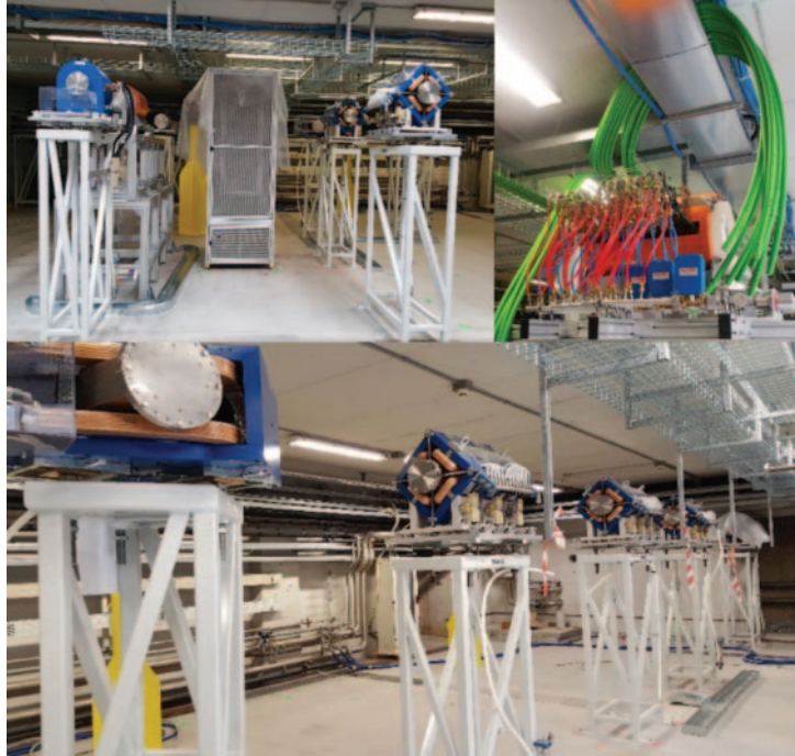
Fig. 5. – The ADIGE Installation phase. Top left: transport line towards the MMRS. Top right: Cabling the Charge Breeder. Bottom: n^+ transport line towards the RFQ.
