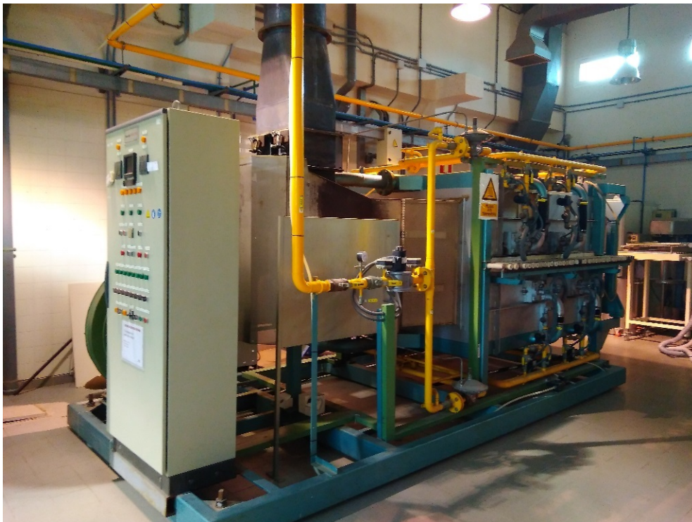
Figure 4: Pilot kiln located at ITC facilities, prior to the installation of the HPHE system.
