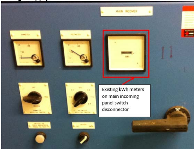
Fig. 3. 400V Switch Disconnector – with legacy kWh Meter
