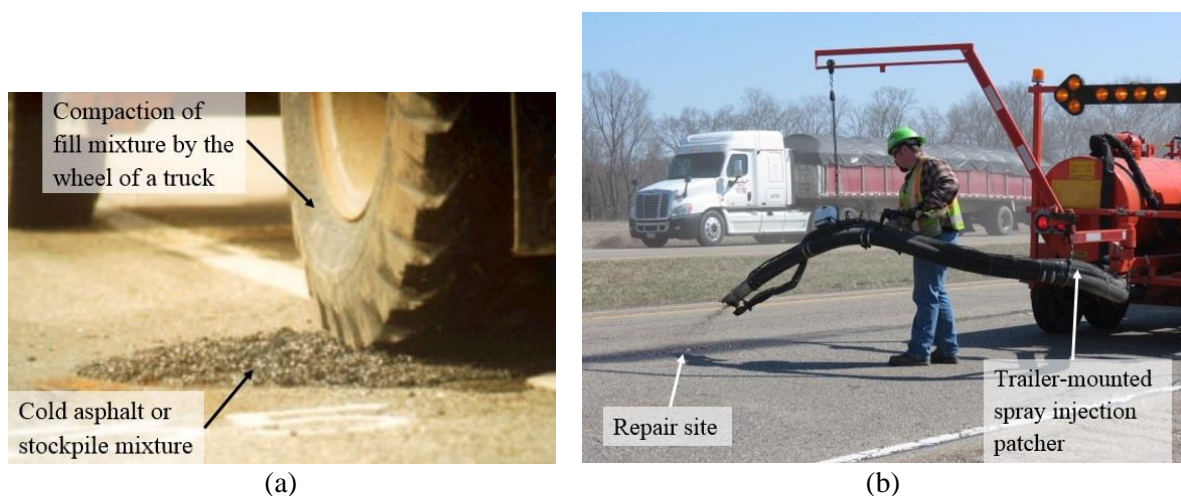
Figure 2.7 (a) Throw and roll; (b) Spray injection repair methods (McDaniel et al. , 2014, (a) p.6 and (b) p.7, label added by author)
