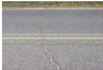
Reflective cracking (Shatnawi, 2008, p.1-8)
