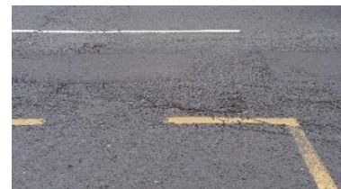
Ravelling or stripping (Uxbridge, London, UK 2016)
