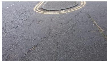
Block cracking (Uxbridge, London, UK 2016)
