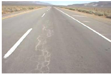
Fatigue or alligator cracking (Shatnawi, 2008, p.1-8)
