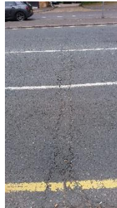
Thermal or transverse cracking (Uxbridge, London, UK 2016)
