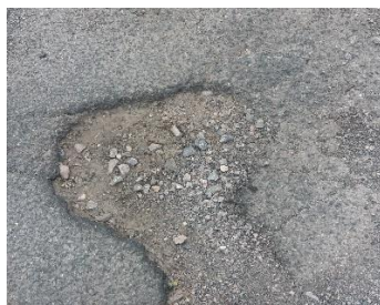
Pothole (Uxbridge, London, UK 2016)
