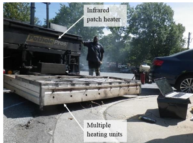
Figure 2.13 Infrared heater used in a field asphalt pavement heating project by Leininger (2015, p.25) (label added by author)
