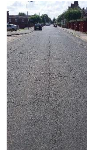
Longitudinal cracking (Uxbridge, London, UK 2016)
