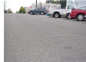
Corrugation (Pavement Interactive, 2018a)
