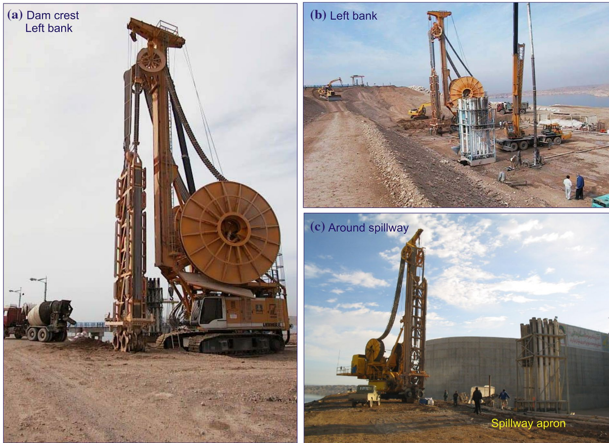
Fig. 4 The BC-40 trench-cutter working at various part of the Karkheh dam during the construction of the complementary cutoff wall
