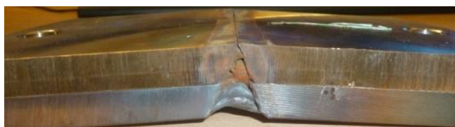
Fig. 15. Welded plates showing residual tensile stress (underneath - inside pipe) and compressive stress (above - outer surface of pipe).
