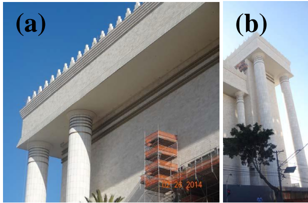
Fig. 2-3 Alkali-activated (a) roof crowning and (b) base and chapter of columns developed by Wincret (Pappalardo, Jalali and Silva, 2014)
