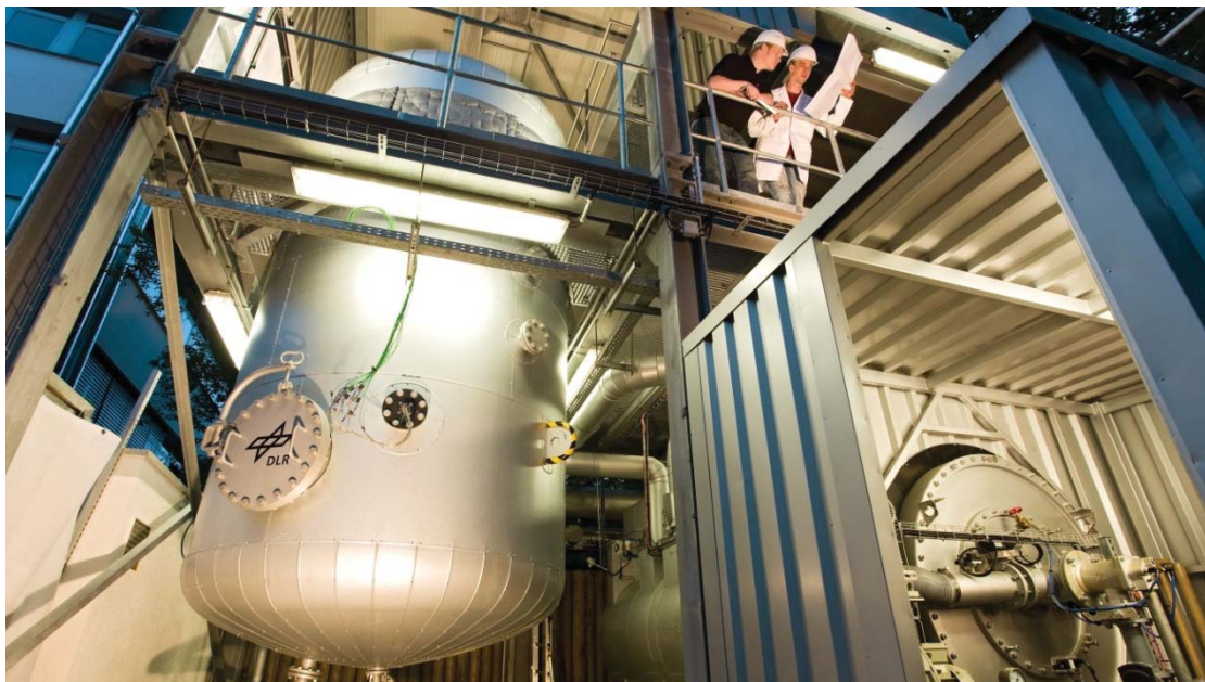
FIGURE 1. Test Facility HOTREG at DLR in Stuttgart
