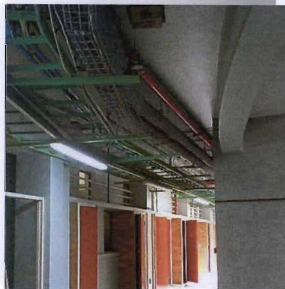
Illustration 5.39: Primary service runs are fixed to a ladder suspended from the passage ceiling. Connections then branch off to work benches from above where required.
