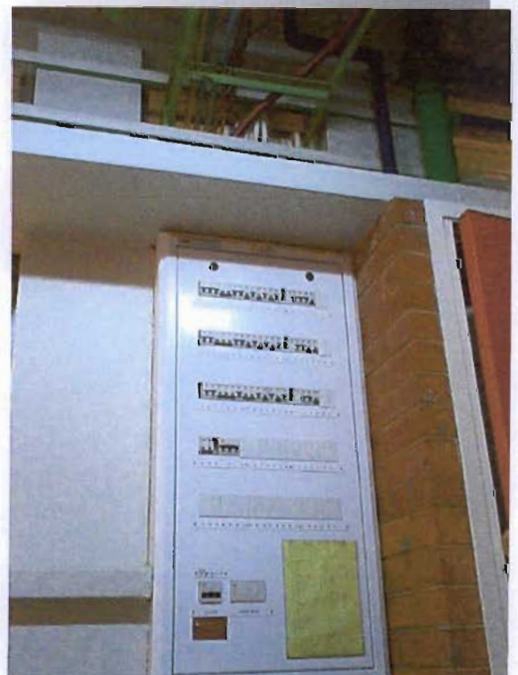
Illustration 7.26: An electrical distribution board outside a laboratory space at the Block H Physics laboratories, Westville campus, UKZN. Notice the spare space for more circuit breakers to allow for future growth of servicing requirements.
