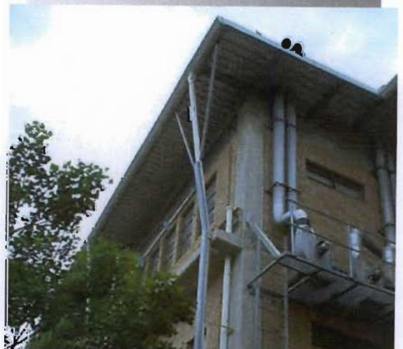
Illustration 5.13: Some additional services attached to the exterior of the building due to the increased requirements during construction.
