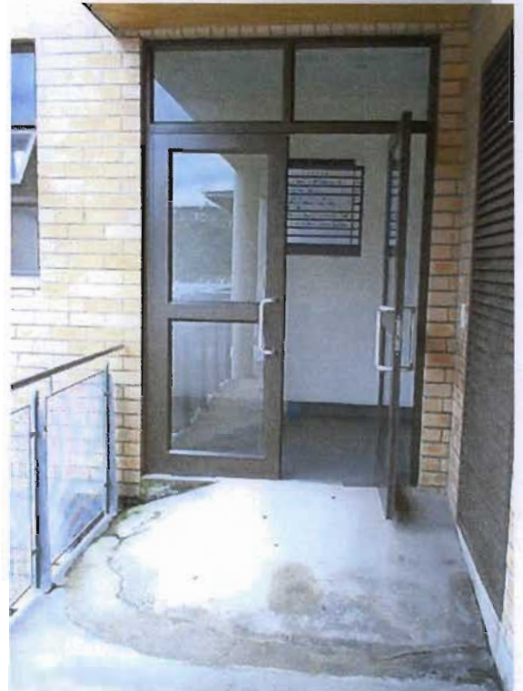
Illustration 5.10: These standard sized double doors, like many other doors in the Institute, do not facilitate the movement of large equipment well. The door should have been full height instead of having fanlights.
