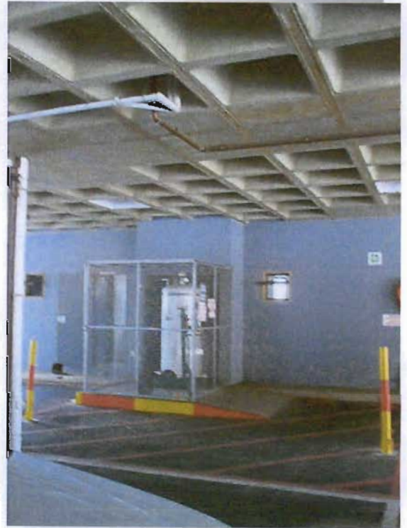
Illustration 5.12: The servicing requirements grew during construction, like many other research institutes, and servicing spaces became inadequate. Some additional service spaces, such as this gas storage area, were placed in the parking area.
