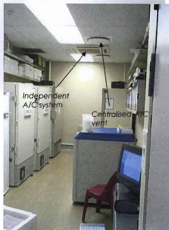
Illustration 5.14 Uninterrupted servicing is crucial in certain spaces. Redundancy systems may be installed such as an independent ceiling mounted A/C in addition to the room being serviced by the centralised system, as shown above.
