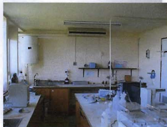
Illustration 5.24: Trunking along a laboratory wall. As initial allocation for services were inadequate, new trunking is run in an ad-hoc manner and consumes otherwise usable wall
