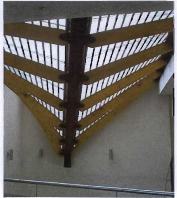
Illustration 5.19: The curved skylight structure over entrance lobby. In a building that has specific practical requirement, creativity can be injected into an ordinary building with elements such as these.
