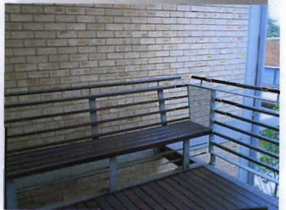
Illustration 5.11: The railings on the balconies are purposefully designed to be easily demountable to facilitate the hoisting of bulky equipment via forklift or crane.
