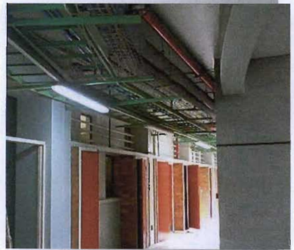
Illustration 7.17: A horizontal service distribution is used in the Block H Physics Laboratories. Service runs are grouped together and run along a service ladder that is suspended from the underside of the ceiling. The system is highly flexible and cost effective.
