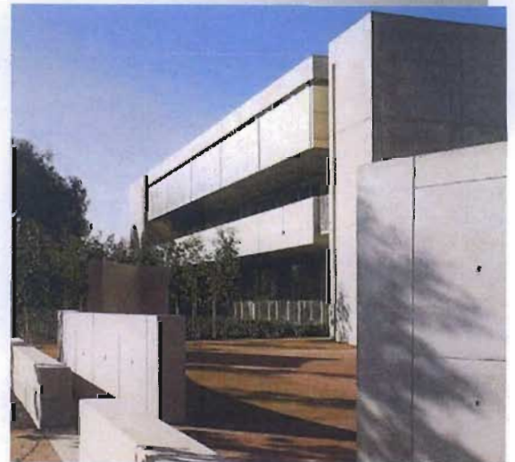
Illustration 4.29: Most of the glazing faces east or west. As seen above, the steel screens shading the west façade of the building do not sufficiently protect the laboratory spaces from direct sunlight in the early morning or late afternoon.
