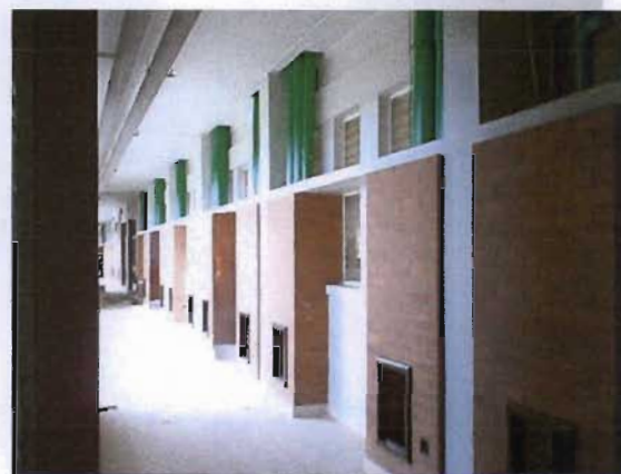
Illustration 5.38: Each group of vertical green pipes indicate a vertical service shaft. This was a popular servicing approach in the past, but has fallen out of favour due to the fire risk it poses.
