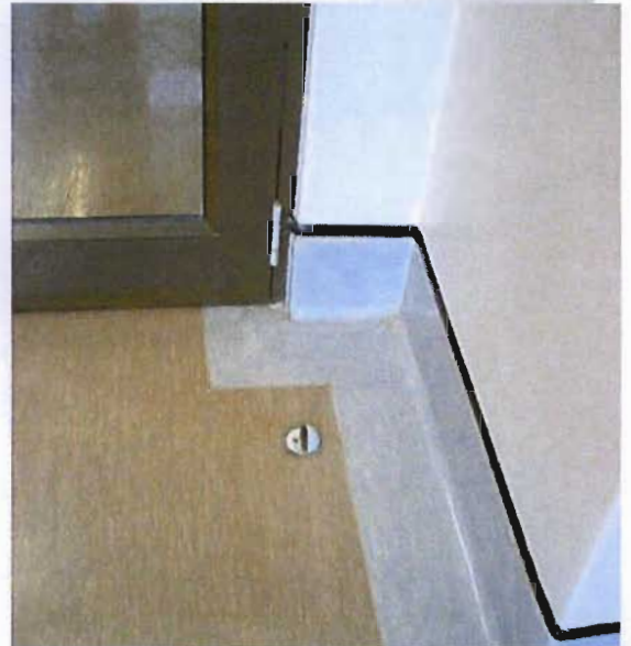
Illustration 5.16: Vinyl sheeting flooring with contrasting coloured skirt. Joints between sheets are torched to create a seamless floor finish.
