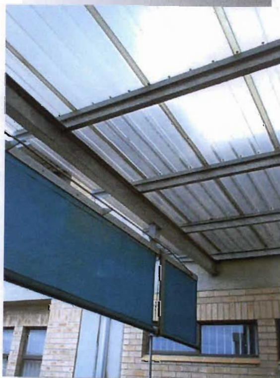
Illustration 5.15: Horizontal screens on the laboratory decks shade the space from the harsh west light.
