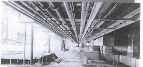
Illustration 4.12: The servicing undercroft. During construction the servicing requirements increased, leading to the undercroft becoming congested. Servicing from below did however result in no structural modification due to change. Source: (Herzberg: 1984, 57)
