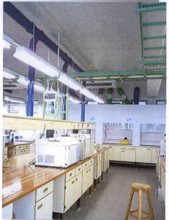
Illustration 5.43: Laboratory benches are serviced from above. The supply branch connects to the primary supply runs that run along the passageway.
