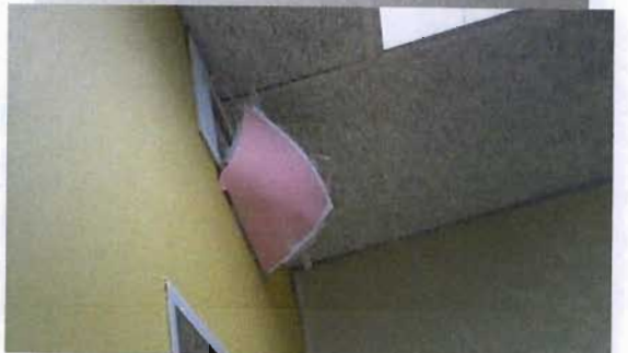
Illustration 5.18: Due to the centralised nature of the A/C system, individual users do not have much control of their environment. Here, the fixed outlet directs air inappropriately and the staff of this office have erected a makeshift deflector.
