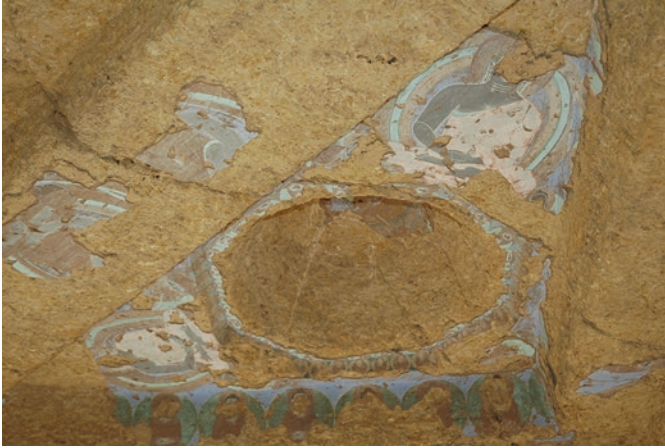
Fig. 8 Intentional looting has resulted in further damage to the few remaining wall paintings at Foladi Cave 4, as seen in severe cutting marks here. (© Y. Taniguchi, courtesy of NRICPT)
