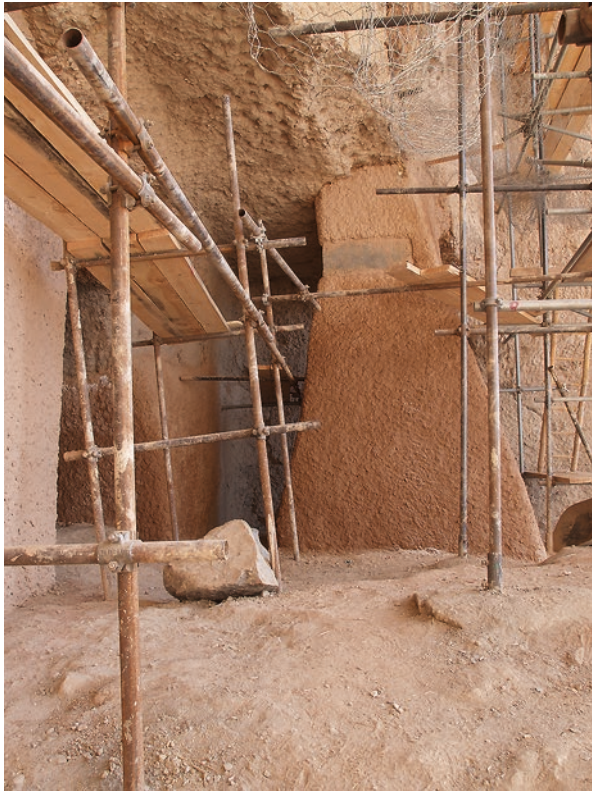
Photo 7 Eastern Buddha, September 2009: reconstruction of cave walls and a pillar at the lower gallery by Erwin Emmerlin, Edwin Fecker and Sekandar Seradj. (© Bert Praxenthaler)
