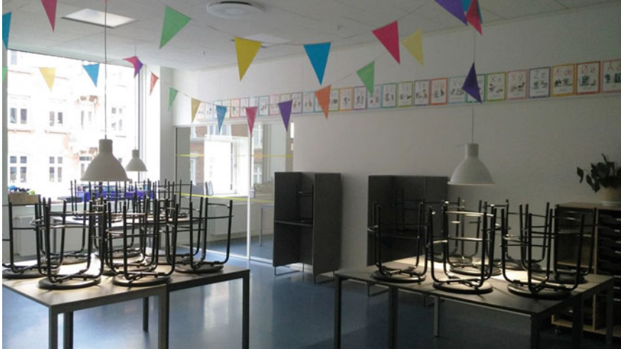
Fig. 7 Permanent lighting installation inaugurated by the pupils and educator. Photo credits: Henning Larsen, Imke Wies van Mil
