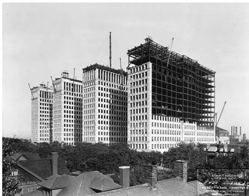
11.5 General Motors Building, Detroit, Michigan, 1923, by Albert Kahn, architect. From the Bentley Historical Library, University of Michigan. Copyright © Albert Kahn Associates.
