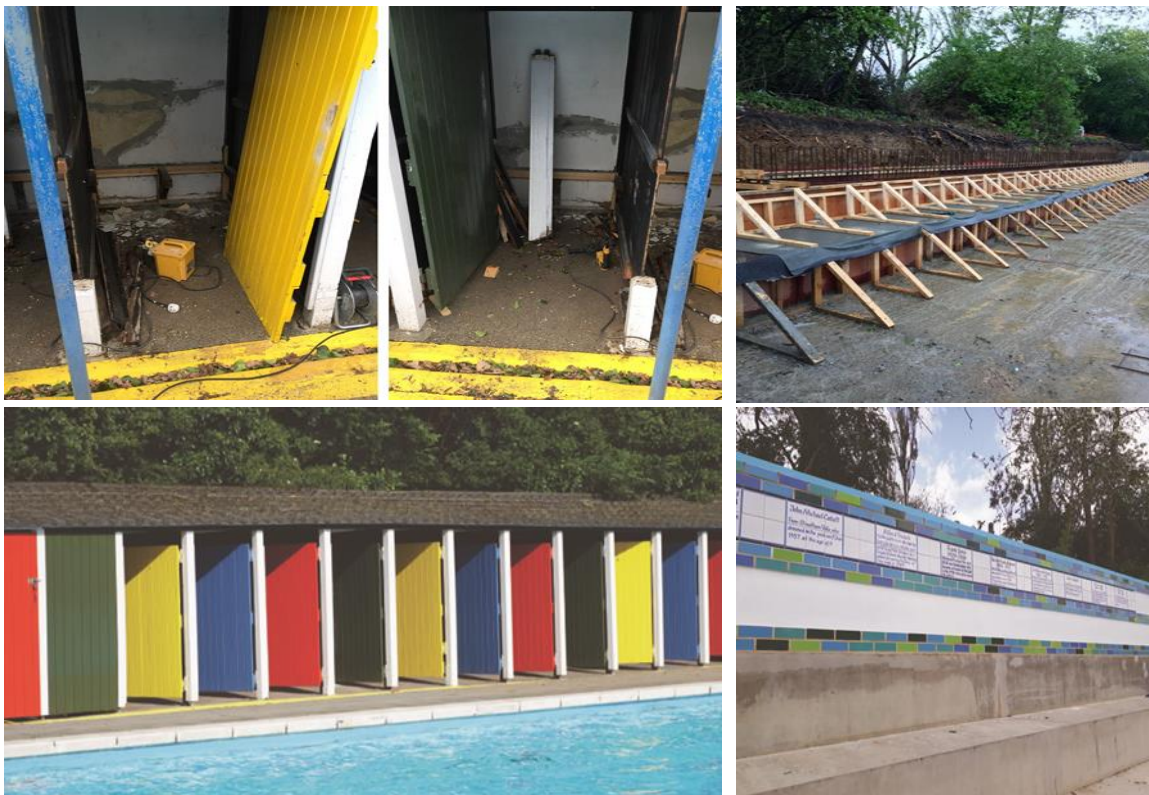
Figure 6 Tooting Bec Lido during works (above) to the cubicles (left) and (right) Western Terrace and (below) completed mid-2019. In addition to commemorating notable individuals associated with SLSC the plaques remember two children who drowned in the pool.
