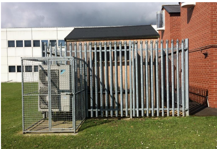
Figure 3-6 Shed with cascade HP. Outdoor unit shown.
