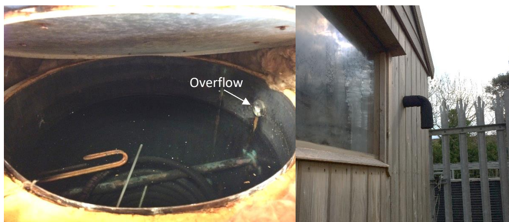
Figure 4-11 Left picture: Inside of thermal store (view from top) with overflow indicated. Right picture: 22mm overflow pipe exiting shed - connected horizontally to thermal store.
