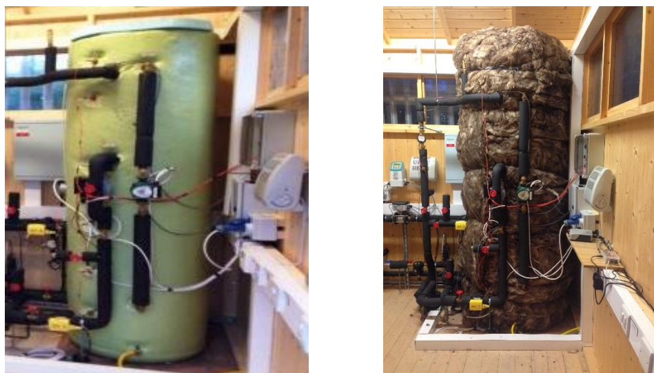
Figure 3-8 Left (A): thermal energy storage tank installed with factory 50mm spray foam insulation. Right (B): thermal energy storage tank installed with additional 100mm glass fibre insulation.
