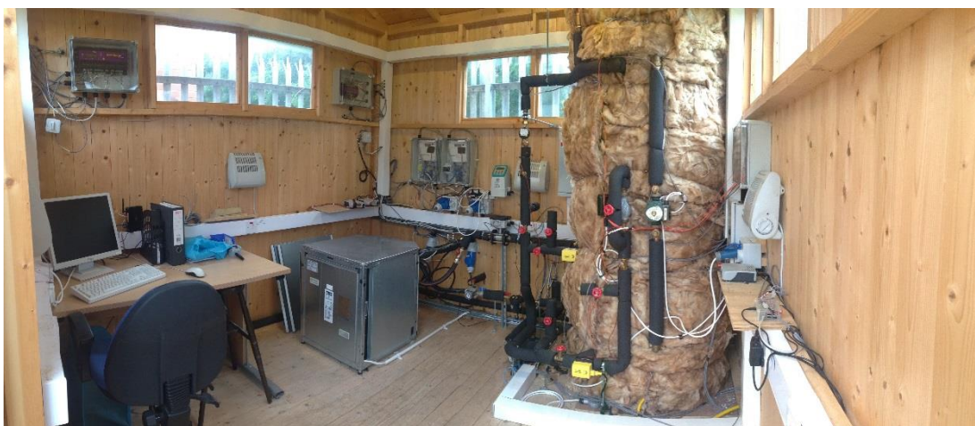
Figure 3-7 Retrofitted cascade HP. Indoor HP unit and thermal storage tank shown.
