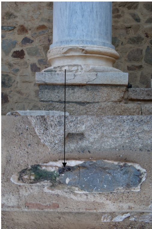
Figure 3. Marble fragment from the basement of a column in the Front Stage of the Roman Theater in Mérida. The degradation of the epoxy resin is visible in both sides of the fracture. (Source: Consorcio de Mérida).
