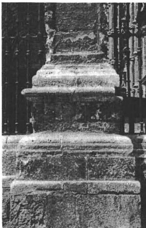
Fig. 2: Limestone wall and pilasters, severely deteriorated due to black crust formation.
