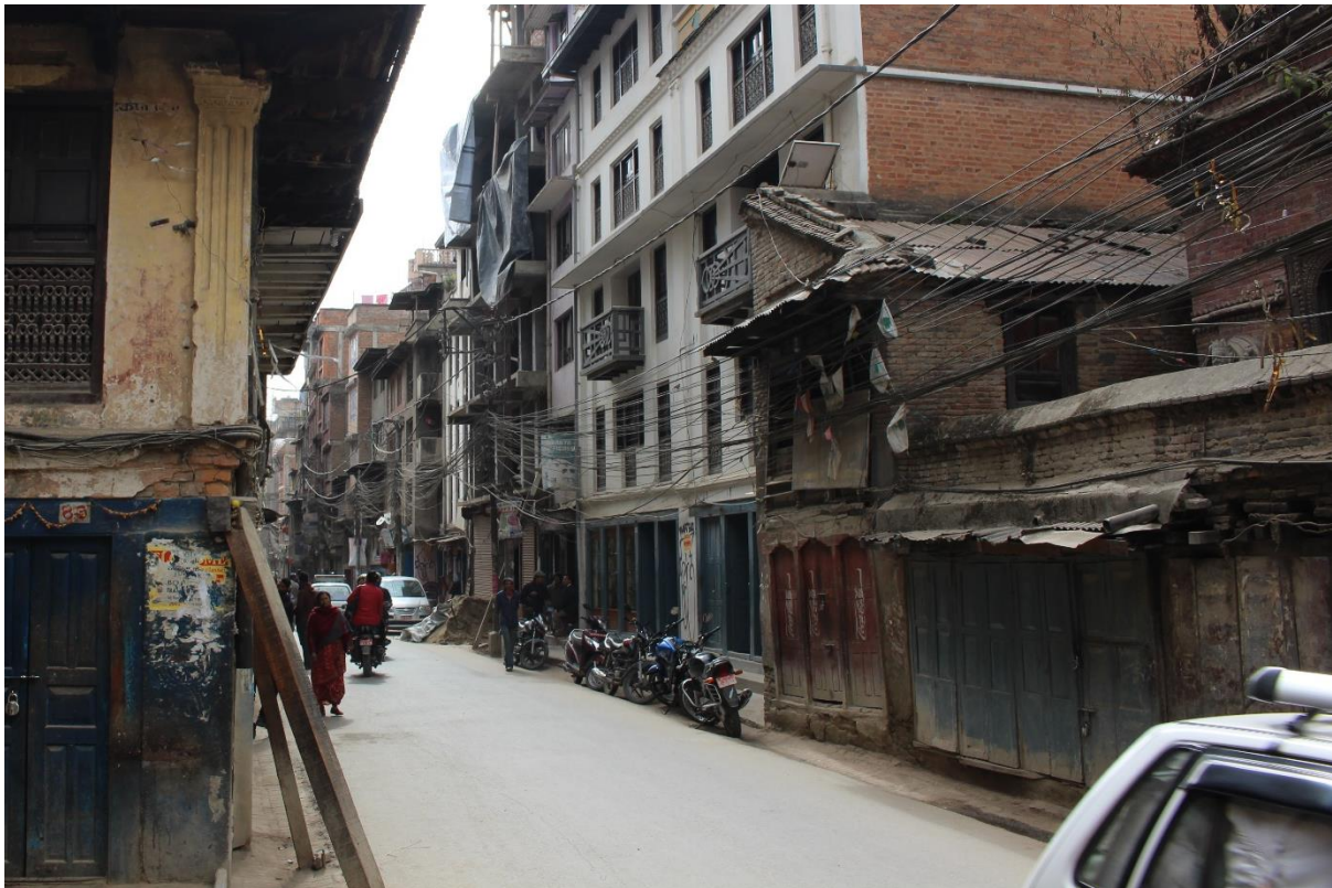
Photo 1: Example of distribution lines attached directly to buildings in Kathmandu. Collapsing buildings in the earthquake damaged lines connected to buildings in this way.
