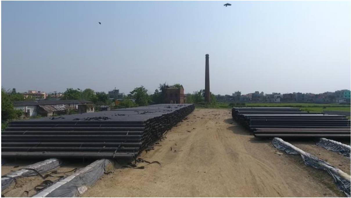
Figure 6.4a: Pipes which will be used for the pipeline connecting the IOC and NOC depots. From NOC (2018e).
