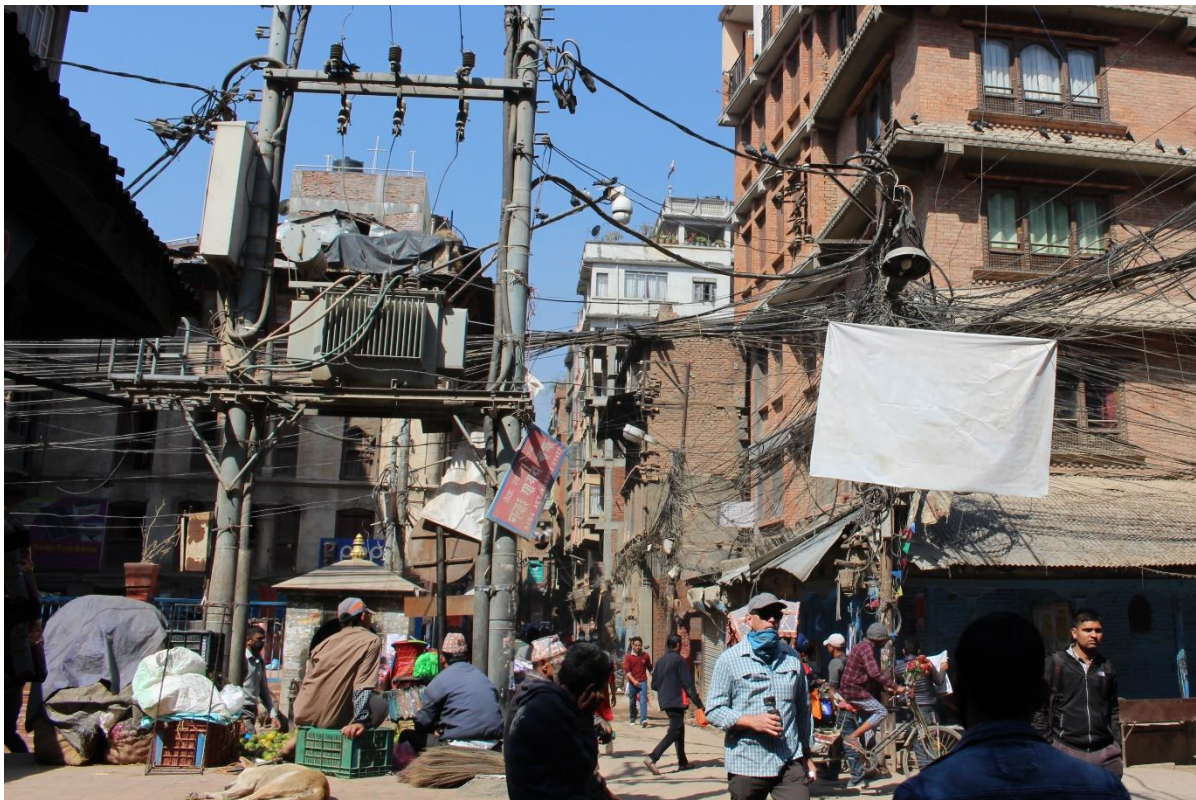
Photo 6: Transformer within Kathmandu's distribution system. Increasing the capacity of this system is an ongoing issue.
