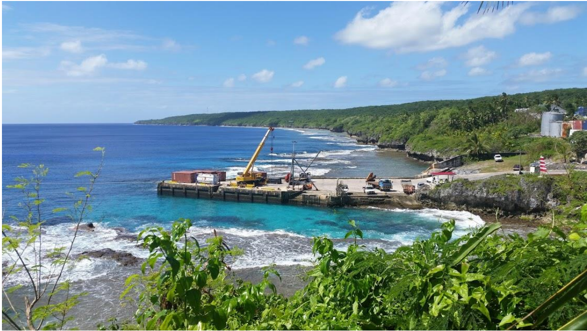
Figure 6.4: Wharf at Alofi busy with loading and unloading containers from the cargo ship (Source: Author, 2018).
