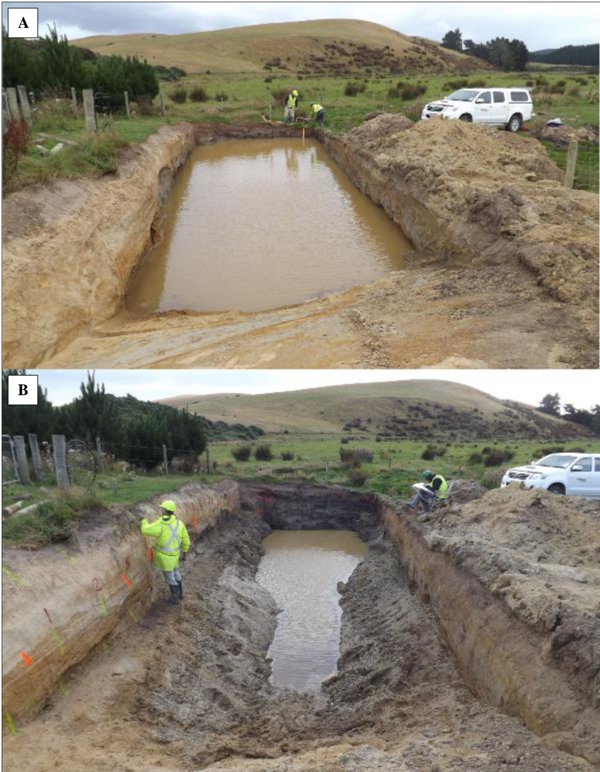
Fig. 2.12 Preparing Rocky Valley trench for logging (facing south-west). A. On arrival the trench was completely filled with water. B. Hours later, the majority of the water was pumped from the trench and the south wall was divided up into 1 x 1 m quadrants.
