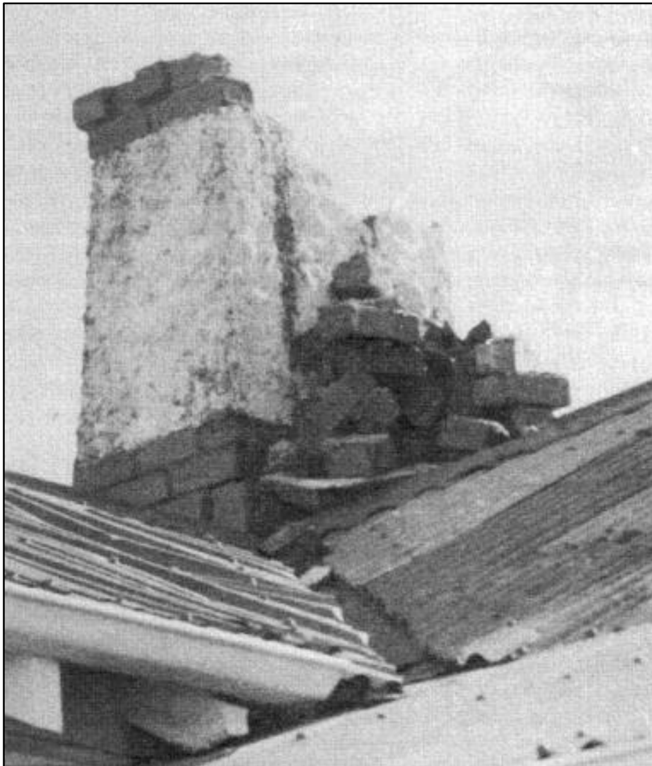
Damaged chimney on house in Bayview Road, Saint Kilda, caused from the 1974 Dunedin Earthquake. Source: Bishop (1974a)
