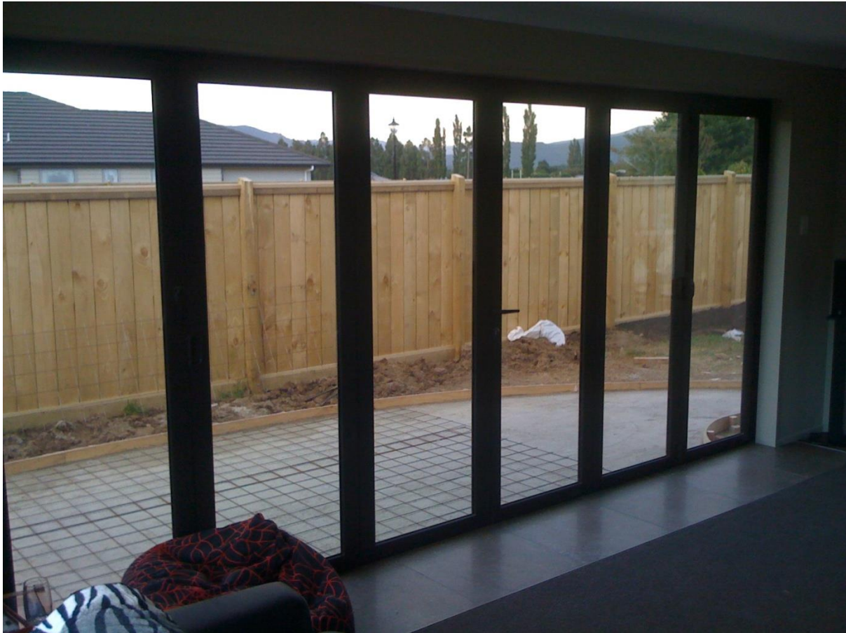
Figure 16.2 Large French doors with tiles inside and out to act out passive solar capture (taken from house 4, the same design as House 1)
