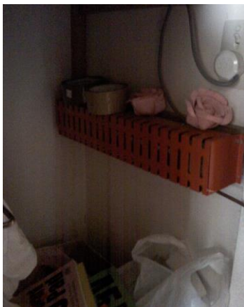
Figure 0.8 Bar heater in laundry cupboard, below hot water cylinder.
