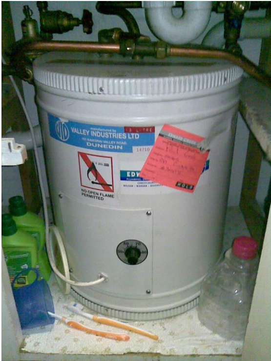
Figure 0.3 The small hot water cylinder, under the kitchen bench
