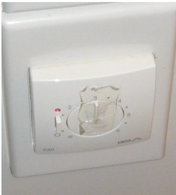
Figure 19: Case 9 under floor heating dial, taped to a specific temperature
