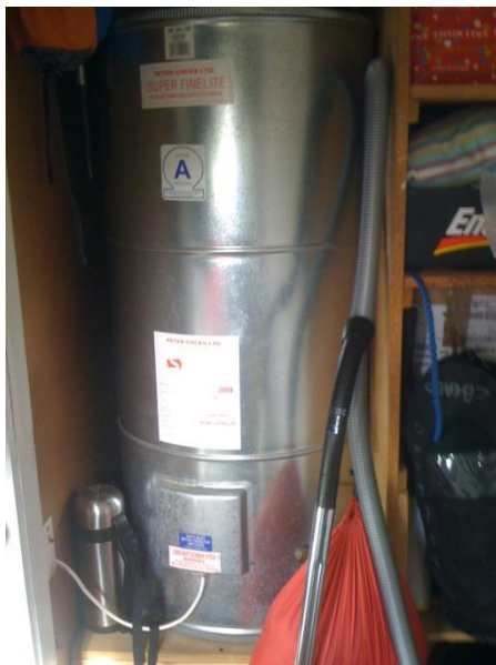
Figure 18: A common electric hot water cylinder in New Zealand (Isaacs, Camilleri, French., 2007)
