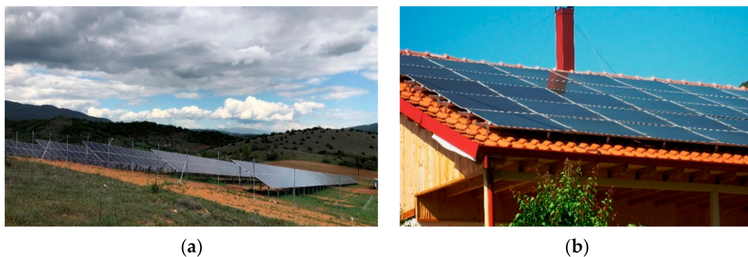
Figure 1. (a) Arnissa ground-mounted photovoltaic farm; (b) One of the five roof-mounted installations of 10 kW capacity.
