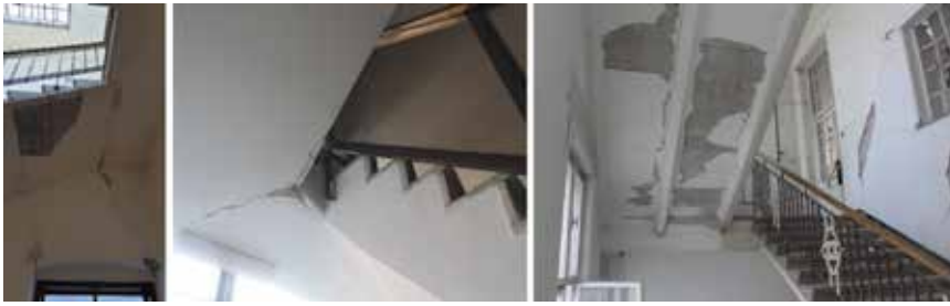
Figure 25. Cases of staircase damage [39]
