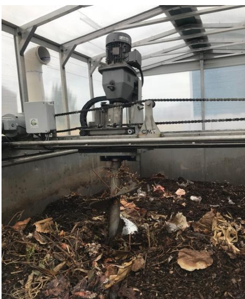
Fig. 8. USU Industrial Food Waste Composting Unit
