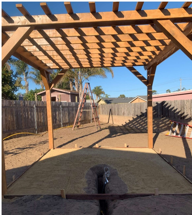
Figure 3: Pergola is built. Border for hardscape and base is set. Waiting on pressure test of gas line to backfill trench and compact decomposed granite.
