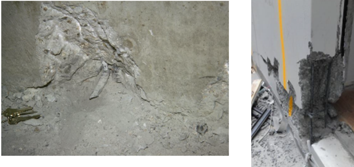
Figure 2-2: Fracture of Longitudinal Reinforcement in Major Earthquakes (Left) Longitudinal rebar fracture following the 1971 San Fernando Earthquake (Birely, 2012) and (Right) Longitudinal rebar fracture following the 2011 Christchurch Earthquake (Kam et al., 2011)
