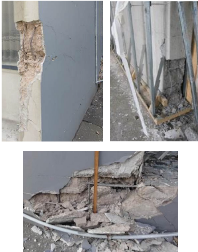
Figure 2-1: Compressive Boundary Element Damage in the 2011 Christchurch Earthquake, Kam et al. (2011)
