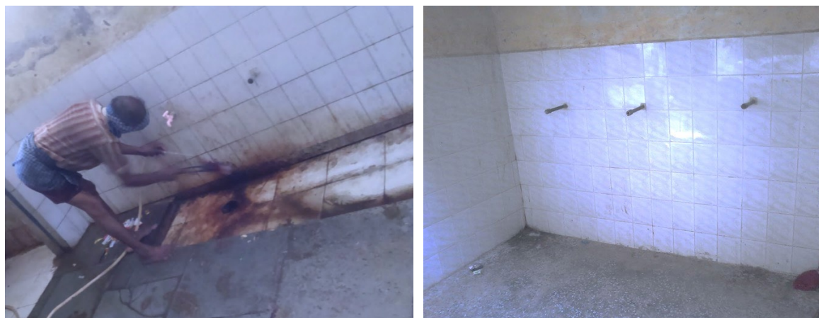
Figure 1: Example of before and after a deep cleaning of a CT in Lucknow
