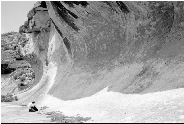
Fig. 2. Photograph showing a typical rock overhang. The rock surface protected from rain and runoff under the overhang is completely covered by the yellowish-brown calcium oxalate coating, while a dark stain (black) occurs on surfaces exposed to rain and runoff.
