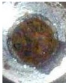
Picture 4. Annulus vent path blocked with corrosion product.
