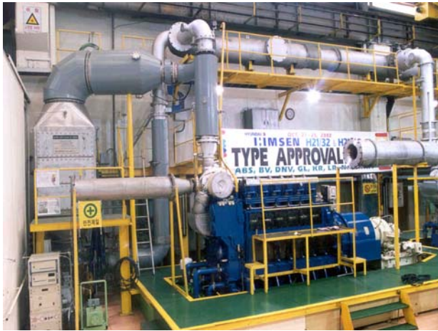
Fig.1 Installed SCR system in Hyundai HiMSEN engine
