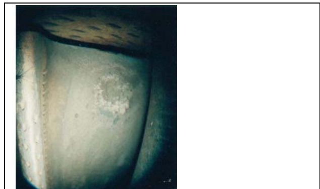
Figure 9: Typical Stage 1 BC-23 Coated Blade After 8,689 Hours (HMAS DARWIN (left) and BC-22 after 7,192 (right) Hours of Operation (CG-52)
